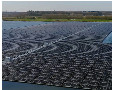
Floating solar farm in Zwolle
